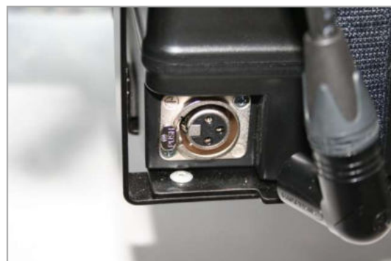
Figure 159: Disconnected plug connection
